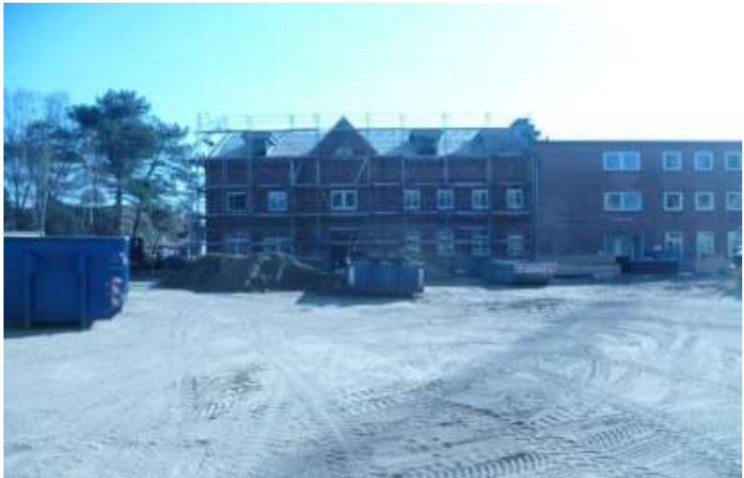
View: the national monument building 24, the entire building is being renovated, and the facade wall refurbished.
